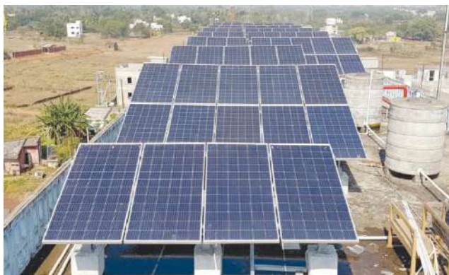
Solar cell in the campus
